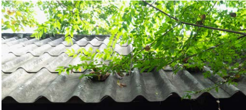
✗ Overgrown trees can cause roof damage.
