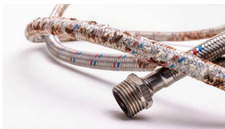
✗ Flexi hose in poor condition.
